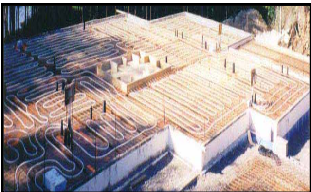
Hambro with Radiant Tubes
