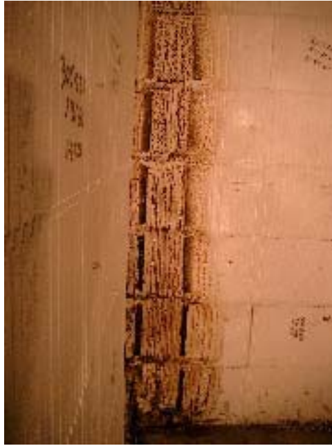
Test Sample After Removal of All Gypsum Wallboard, Right Wall
