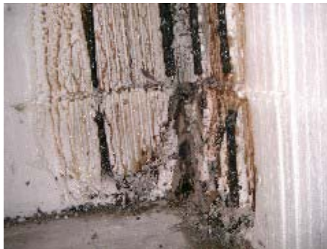
Test Sample After Removal of All Gypsum Wallboard, Crib Area
