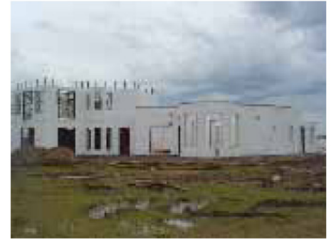
Reinforced concrete inside ICF walls are so much stronger than wood frame that designers can add features, such as the large series of windows on this Knights Ferry California home, that would not be possible with other construction methods.
